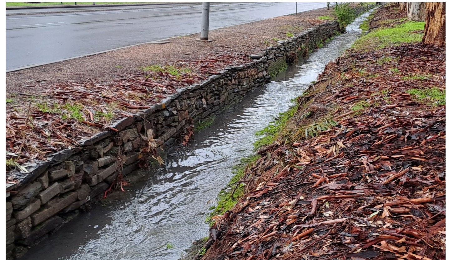
Stacked stone and concrete slab retaining wall with unsafe sheer drop into channel
